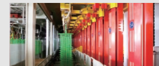
Hanger Electroplating Department
