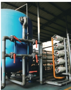
HSD Cambodia Factory Wastewater Treatment System HSD柬埔寨工厂污水处理系统
